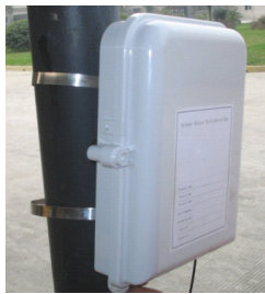
fiber termination box on the pole
