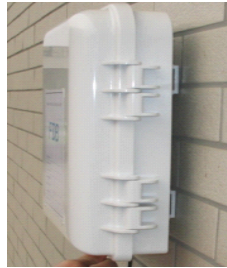
fiber termination box on the wall
